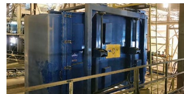
ATLAS units in the production of Frac Sand
